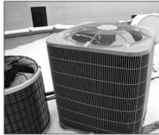
Air conditioning systems
